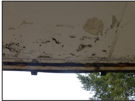
Left: Crumbling ceiling observed at an Albany County shelter in February 2016. Right: The same ceiling condition observed in March 2019.
